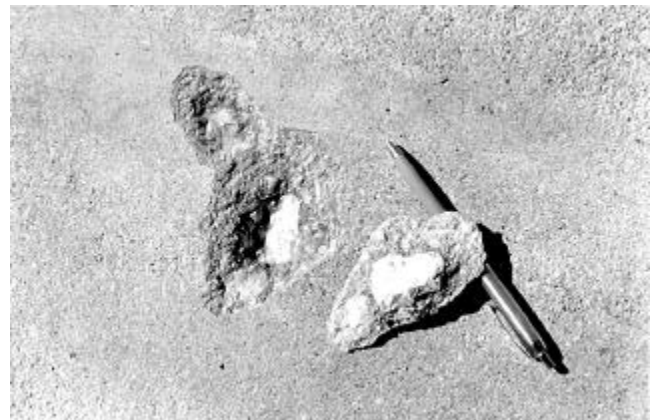
Fig. 11.6—A popout is a small fragment of concrete broken away from the surface of a slab due to internal pressure, leaving a shallow, typically conical, depression
