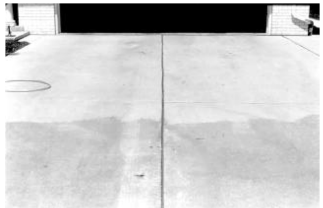
Fig. 11.9—Concrete slab discoloration due to the use of calcium chloride admixture. Concrete in the upper part of the photo did not contain the admixture
