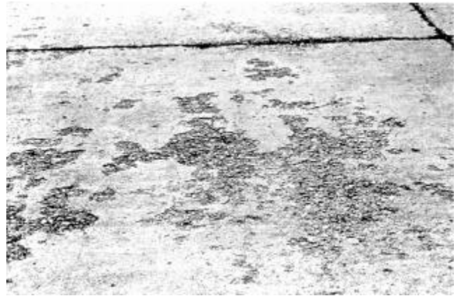
Fig. 11.5—Scaling is the loss of surface mortar, usually exposing the coarse aggregate
