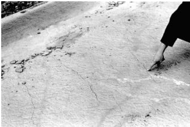
Fig. 11.2.2.1—Plastic shrinkage cracks are caused by rapid loss of mix water from the surface while the concrete is still plastic
