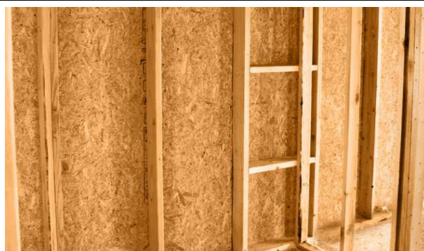
Ladder junctions at interior-exterior wall intersections (Figure 5) produce wall cavities that can be easily insulated to help builders earn the ENERGY STAR® label for new homes.
