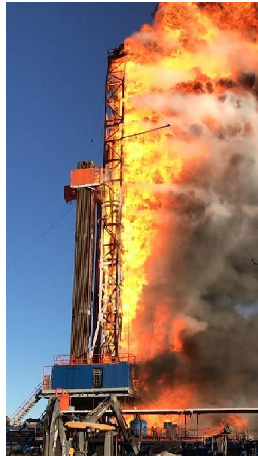
Figure 30. Video still of the blowout and fire taken shortly after it started.
