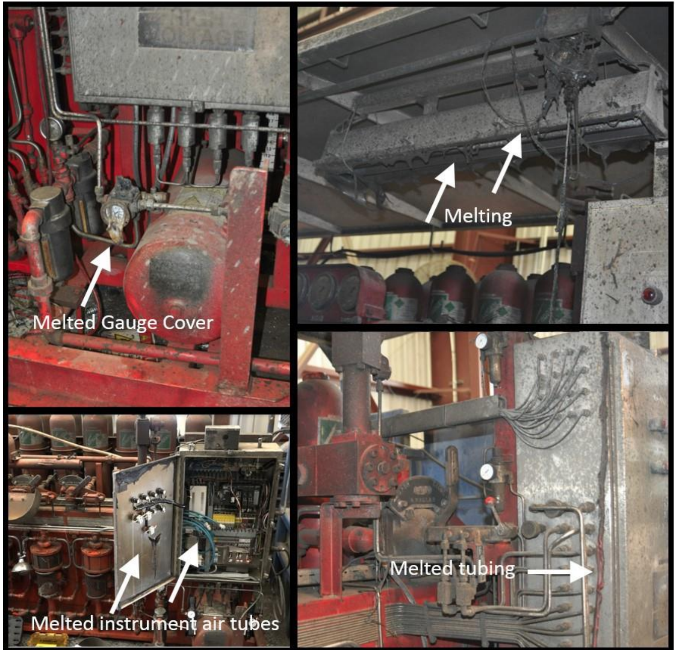
Figure A- 2. Photos of observed heat damage to Patterson Rig 219 accumulator
