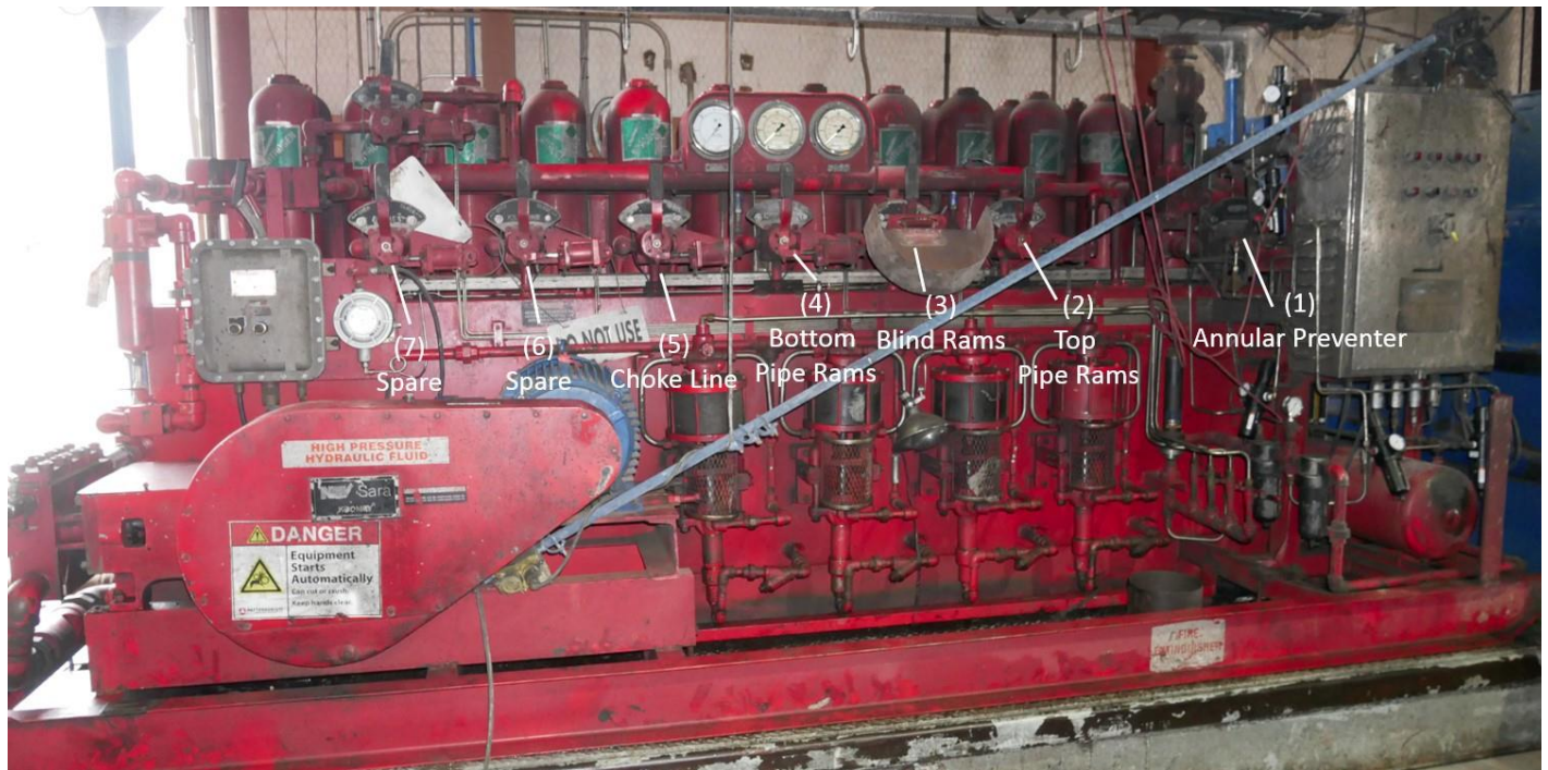
Figure 31. Photo of the BOP accumulator, which is used to function the BOP rams. The rig manager closed the BOP control handles in the following order: (1) annular preventer, (2) top pipe rams, (3) blind rams, and (4) bottom pipe rams. The blowout preventer did not seal the well to stop the blowout when the rig manager functioned the control handles.
