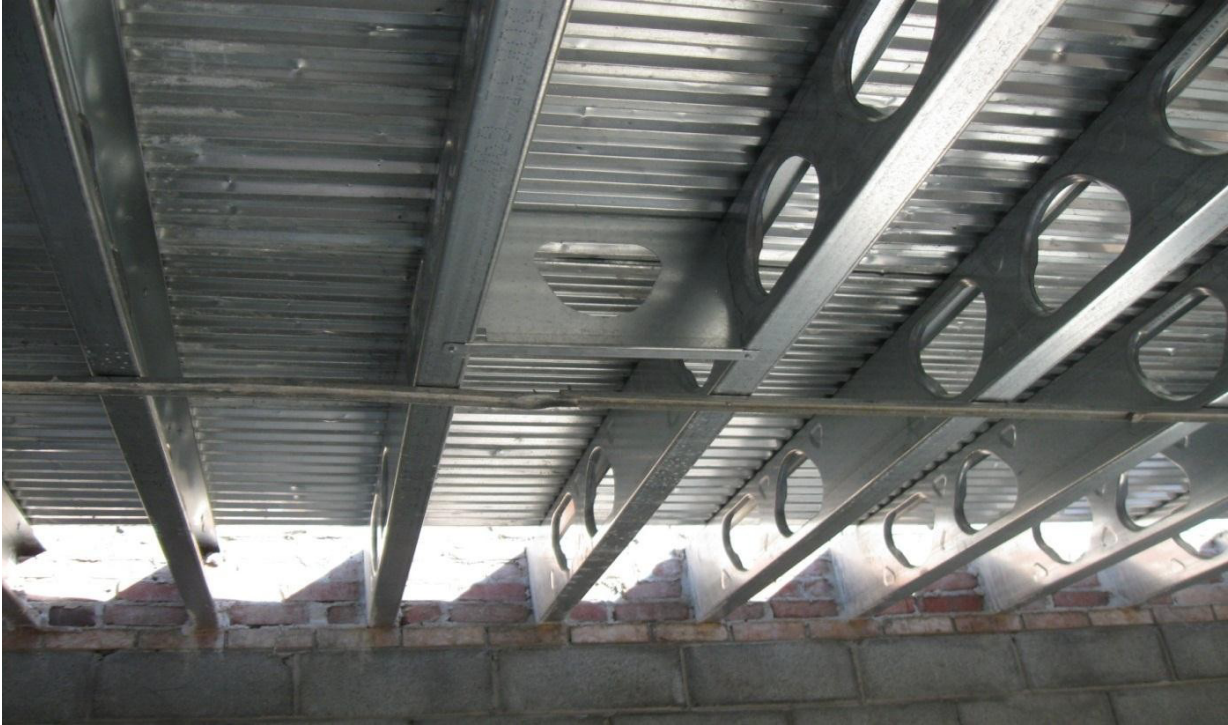
Fig. 4 Floor joists with no straps at the top flange.
