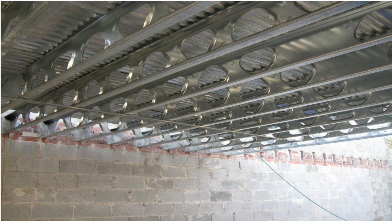
Fig. 5 Floor joists with straps only at the bottom flange.
