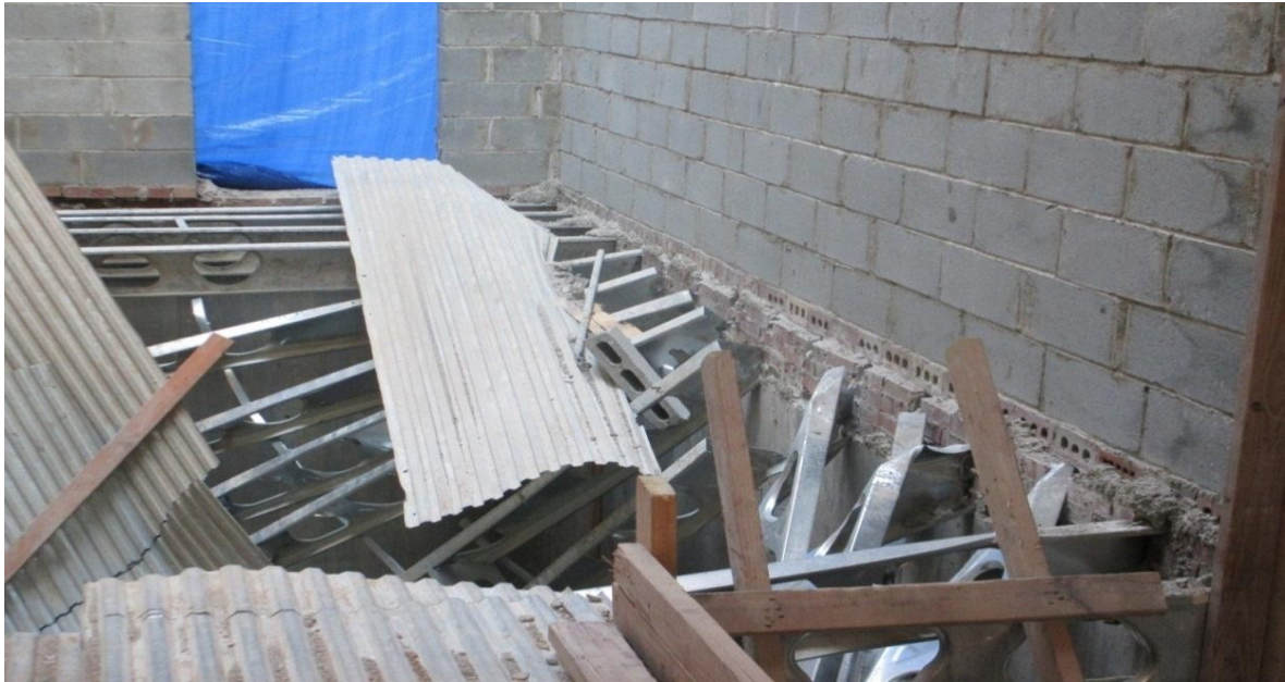
Fig. 9 A partially collapsed 4 th floor due to construction loads.
