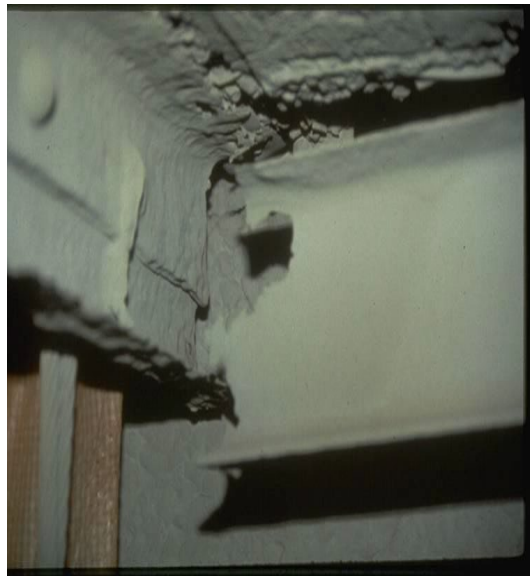
Figure 1. Photo. Photograph of a severed connection due to corrosion.
