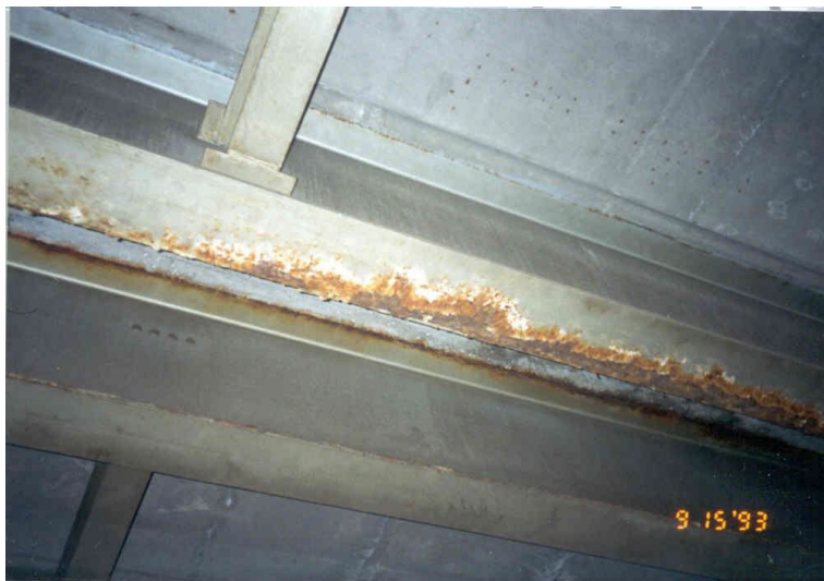
Figure 17. Photo. Steel directly beneath longitudinal expansion joints that have leaked corrosive runoff from the deck.
