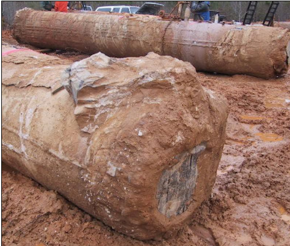
Figure 2.3: Photo of exhumed PGDS showing unintentional flow of grout up the side of the shaft (Brown et al., 2010).
