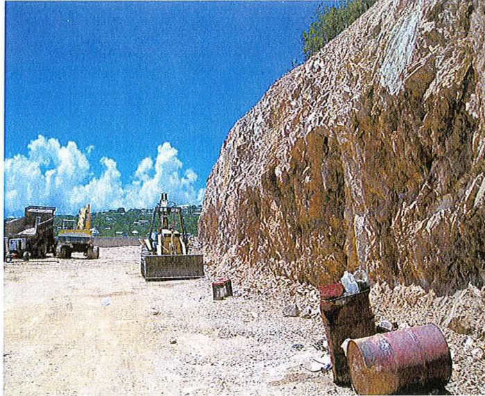
Figure 13. Excavated Surface North of the Collapsed, Looking Toward South.
