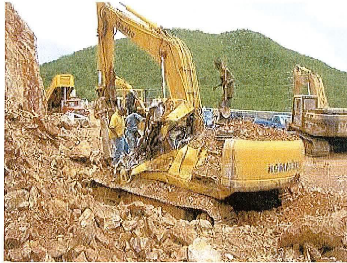
Figure 5. Location of the Komatsu PC 220 Excavator during the Rescue Operation, Looking Toward North (Provided by GEC, LLC.).
