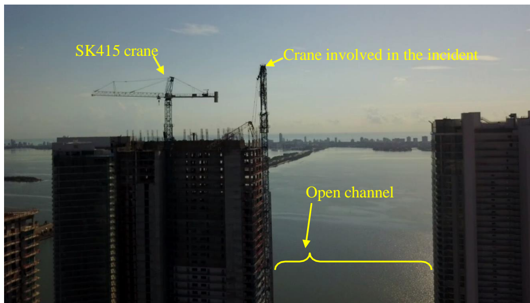
Figure 21 Aerial view of the second failure site – looking east
