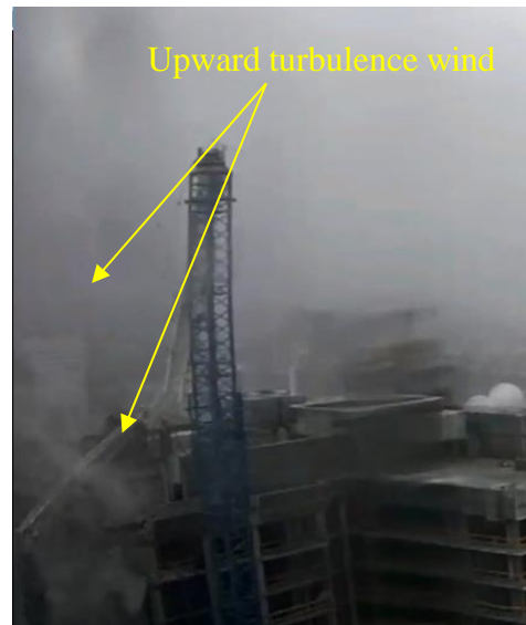
b) Upward turbulence wind detected right after counterweight blocks hit the building
