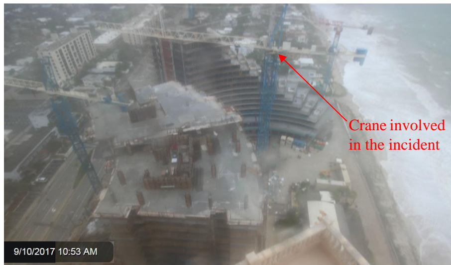
Figure 14 Tower cranes prior to the incident – the third failure site
