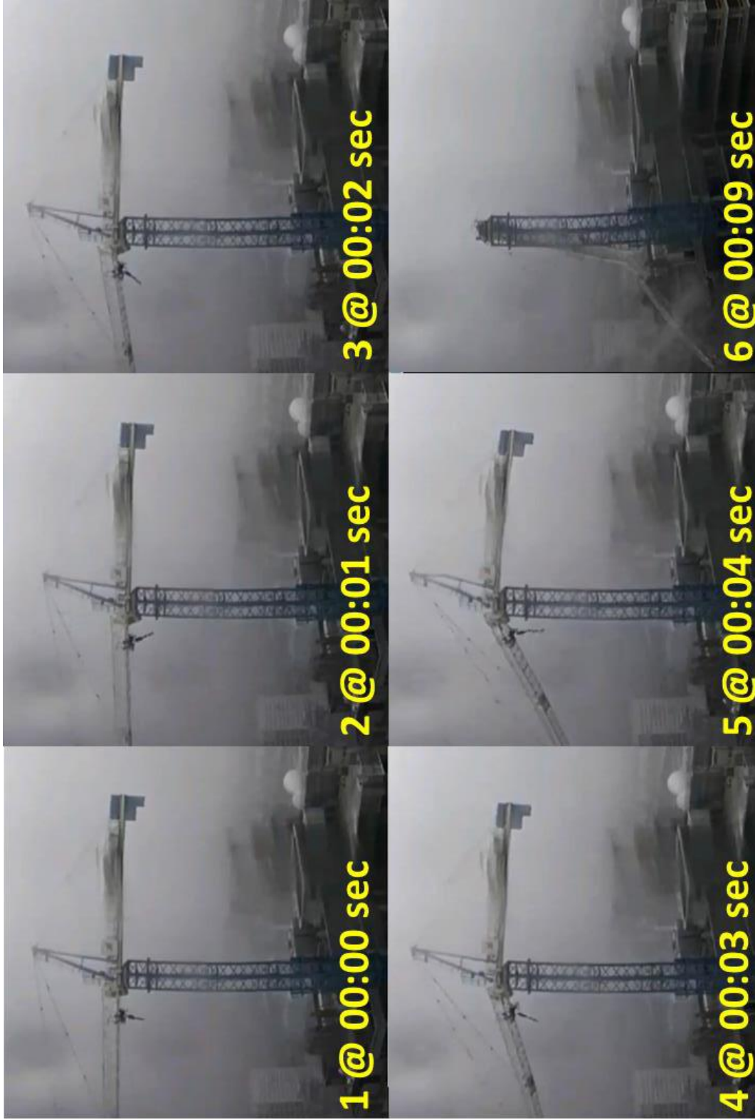
Figure 10 Image sequence showing the crane collapse (Courtesy of Nick Tangredi)
