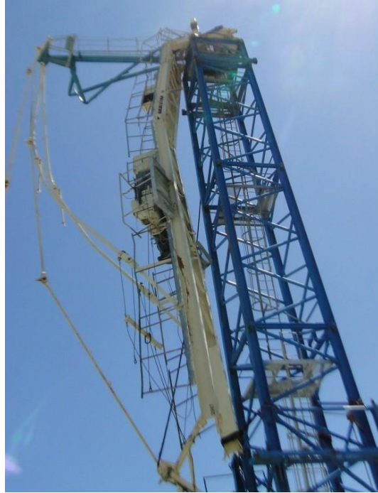
Figure 9 Tower top and counterjib after the incident – the first failure
