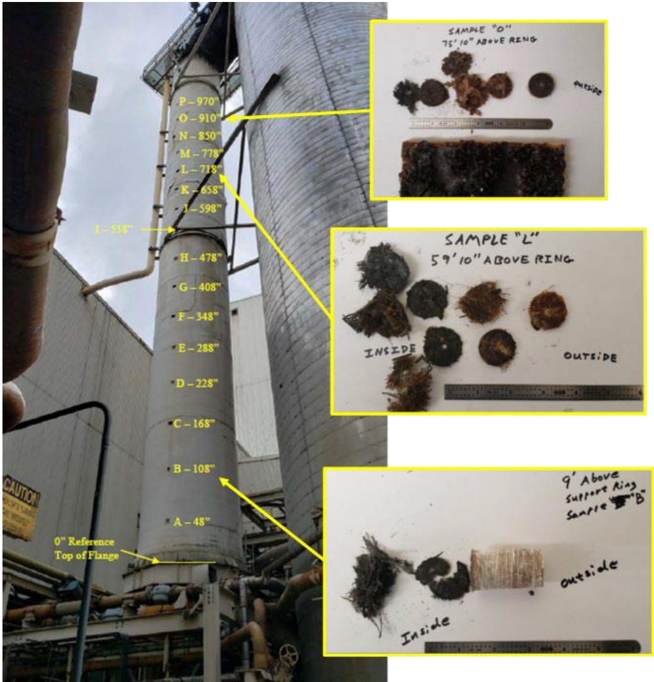
Figure 10. Internal fire damage in the upflow tower. (Credit: Evergreen. Edited by CSB.)
