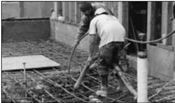
Photo: Richard Parker, 45 © Architects
