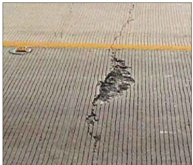
Figure 9. Spalling along transverse crack in a CRCP.
