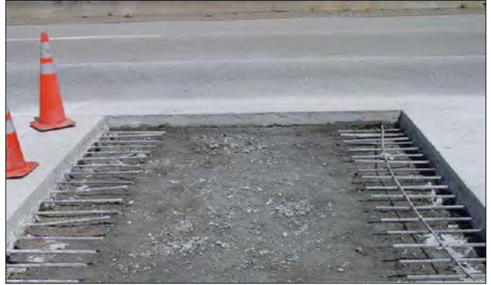
Figure 70. Longitudinal steel exposed in CRCP ready for splicing with new reinforcing steel.
