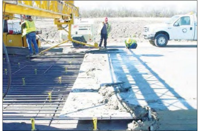
Figure 44. Wooden panels temporarily placed to facilitate removal of concrete carried over end-of-day header.
