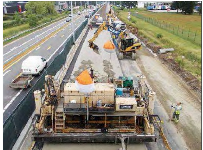
Figure 64. Construction of two-lift CRCP using two slip-form pavers on the A13 roadway (Belgium).
