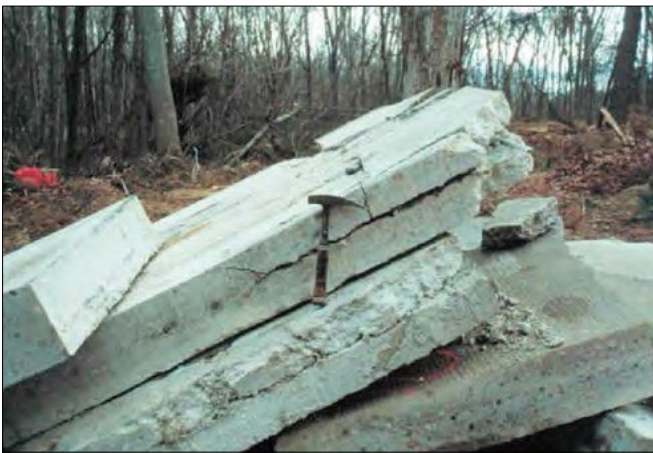
Figure 10. Horizontal cracking plane in CRCP.
