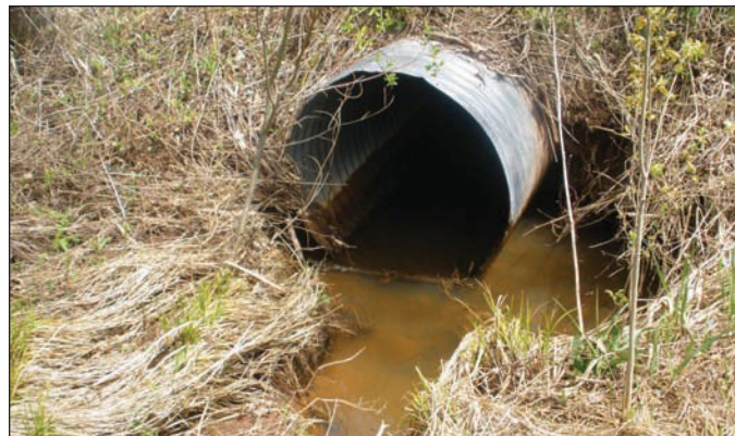
Figure 6: Minor erosion around culvert
