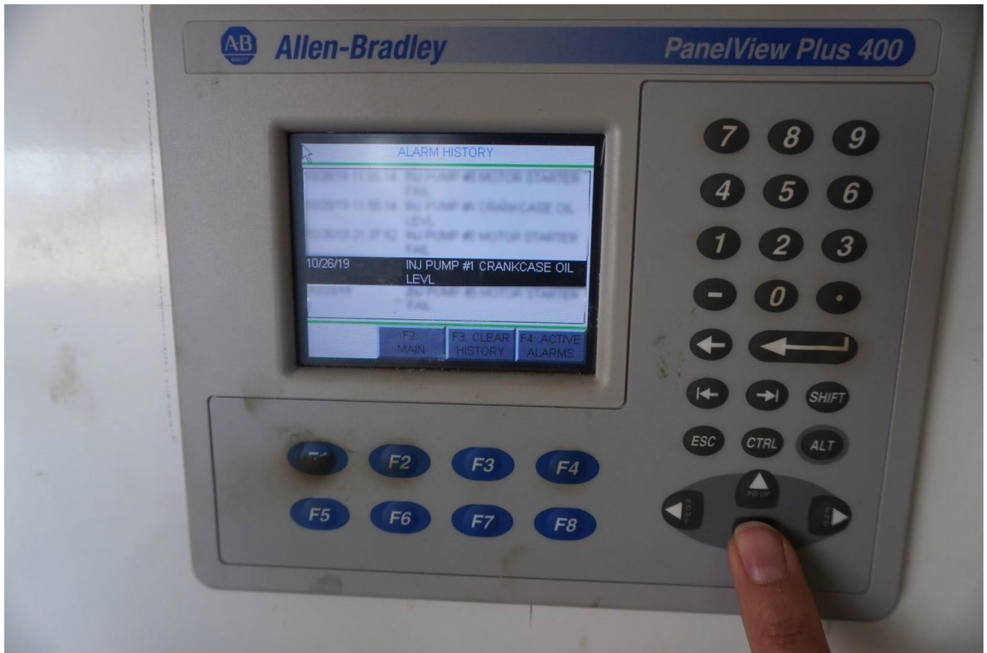
Figure 22. PLC screen displaying Pump #1 crankcase oil level alarm. (Credit: CSB)
