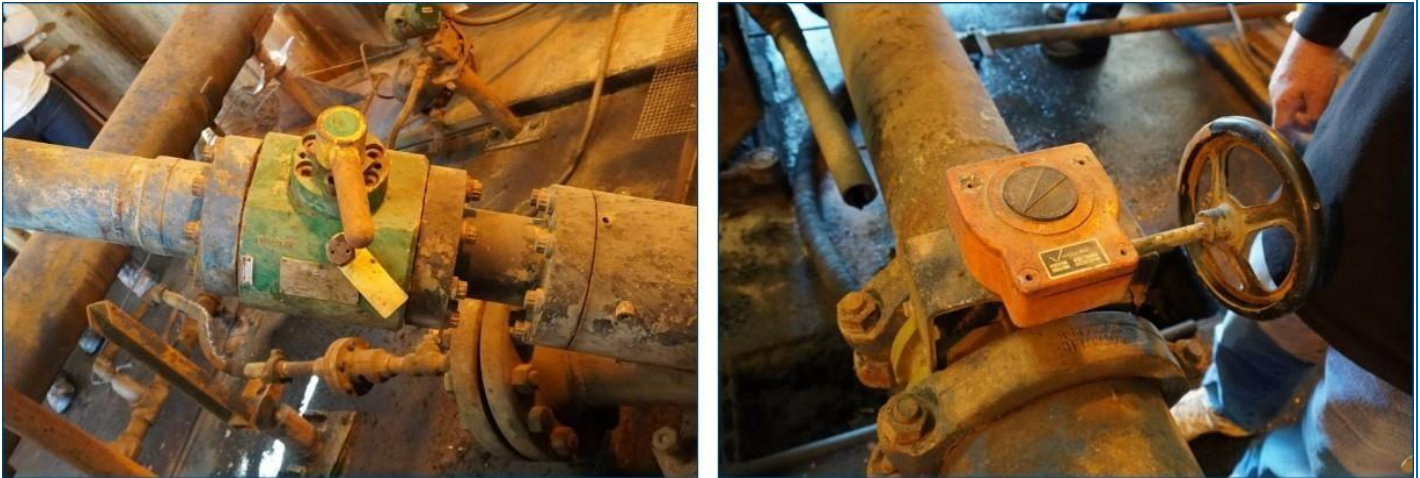
Figure 19. Position of the discharge (left) and suction (right) valves on Pump #1. (Credit: CSB)
