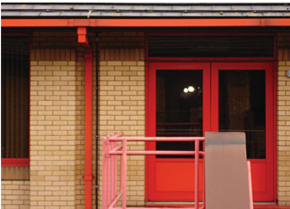
Figure 54. Example of poorly located a down-conductor.
