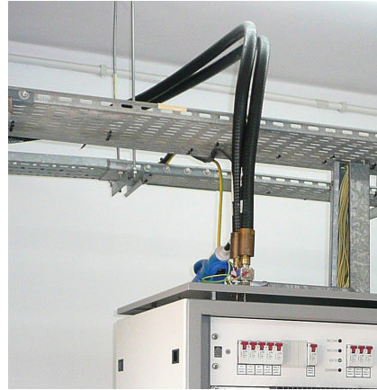
Figure 113. Incoming antenna circuits require protection.
