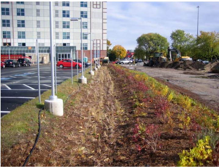
An example of a biofilter in Portland, Maine. (Source: University of Southern Maine, Portland)
