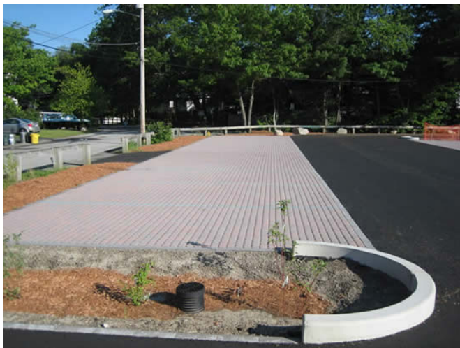
An example of permeable paving. (Source: Silver Lake Project: Massachusetts Executive Office of Energy and Environmental Affairs)
