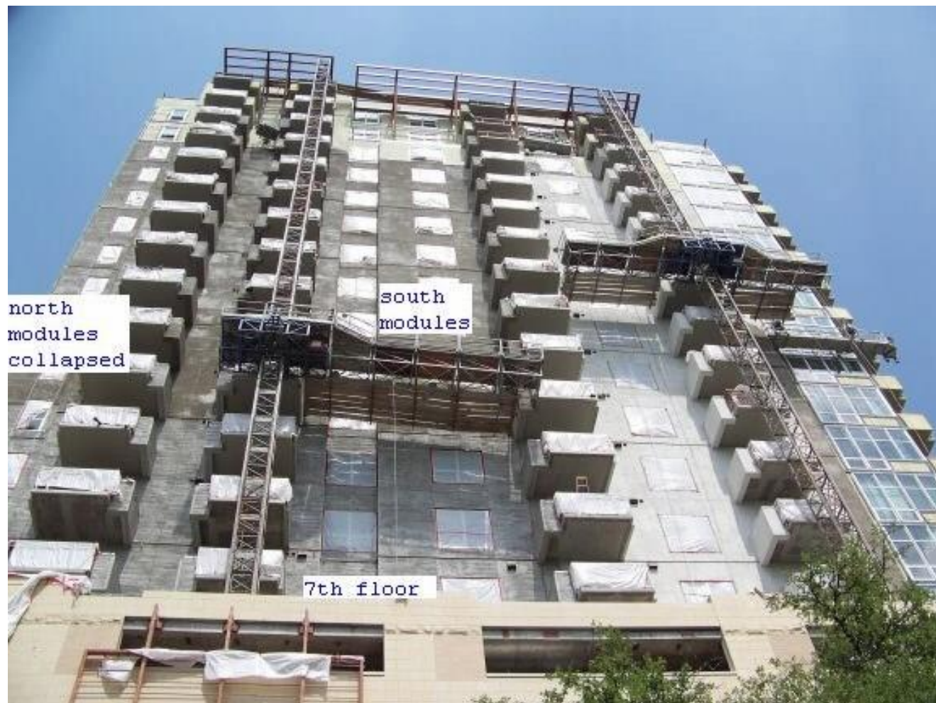
Figure 1 - Failed scaffold with north side modules separated.
