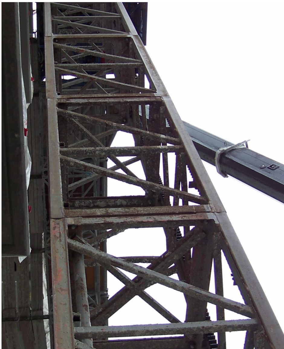
Figure 5 - Tower Mast showing non-uniform and rusted sections
