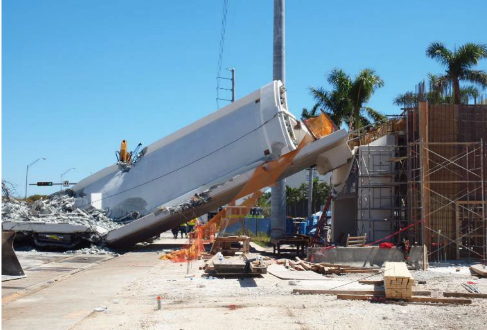
Figure 74 South end of the bridge after collapse – looking east
