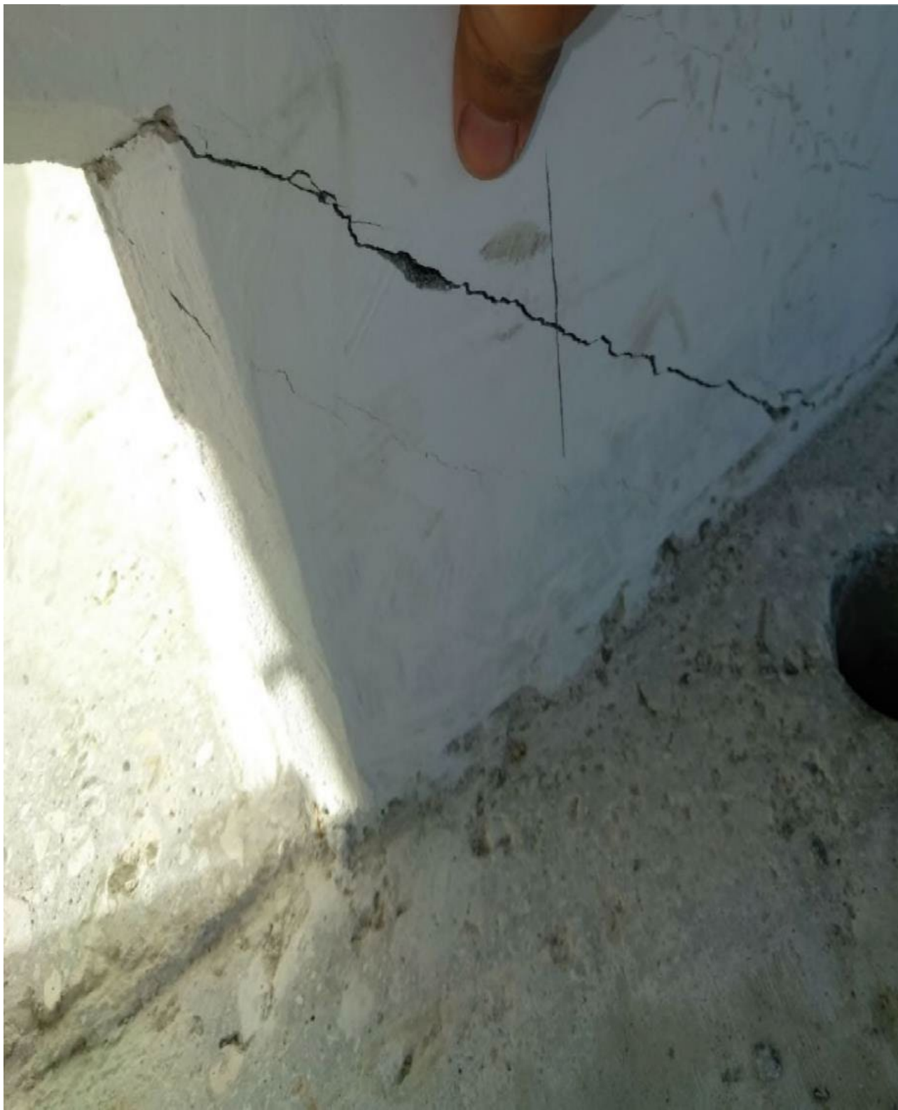
Figure 18 Photo #4 in 2/28/2018 E-mail from MCM to FIGG
