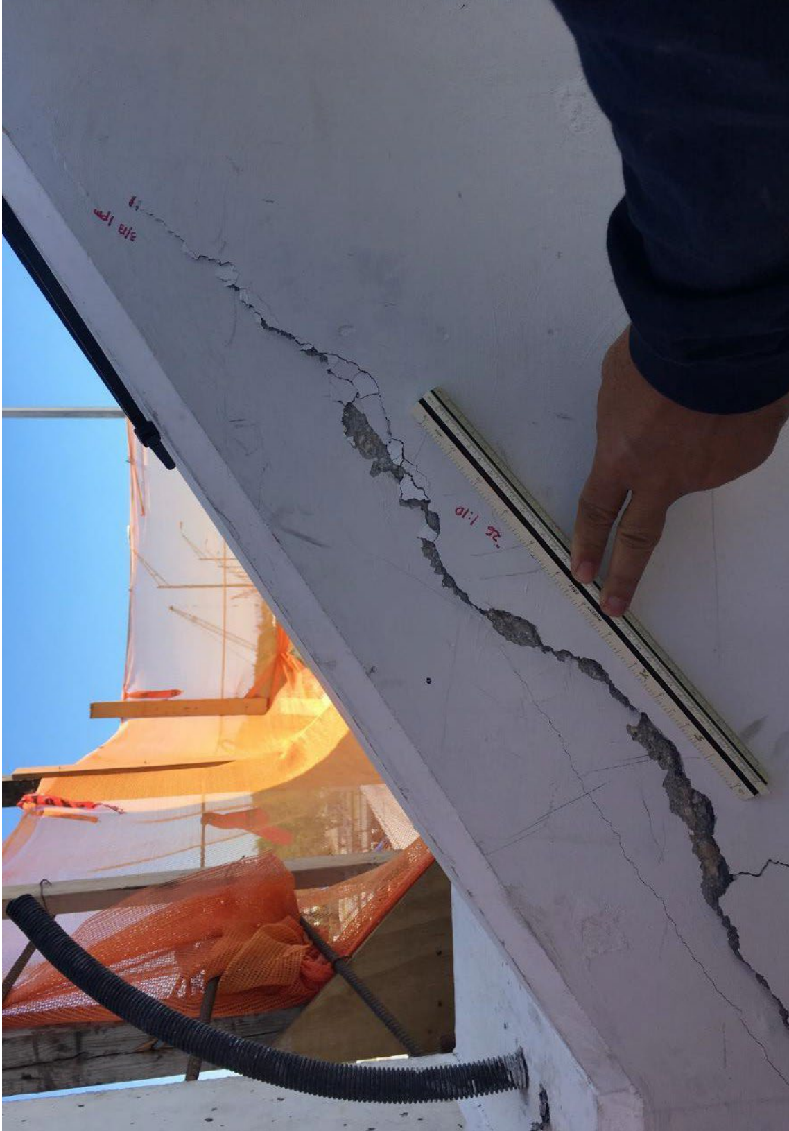
Figure 41 Close-up of longitudinal cracks in diagonal 11 on 3/13/2018 by BPA
