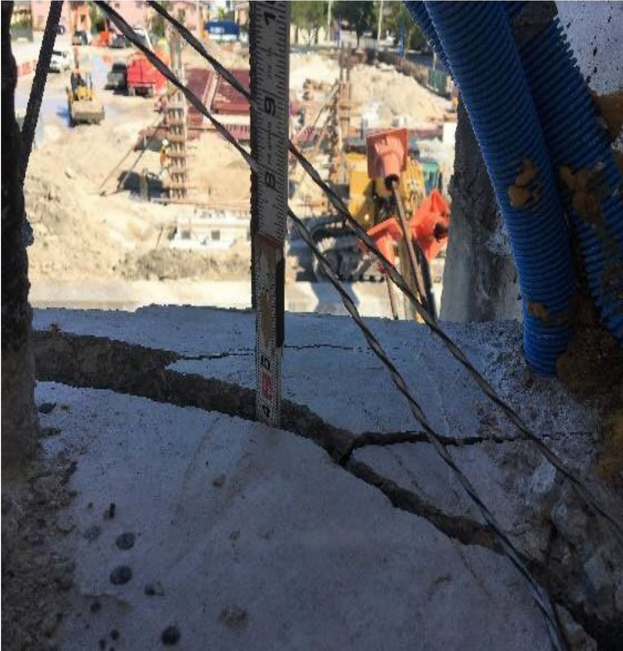
Figure 30 Notice the depth and width of diagonal cracks at the west side of diaphragm II on 3/14/2018 by BPA
