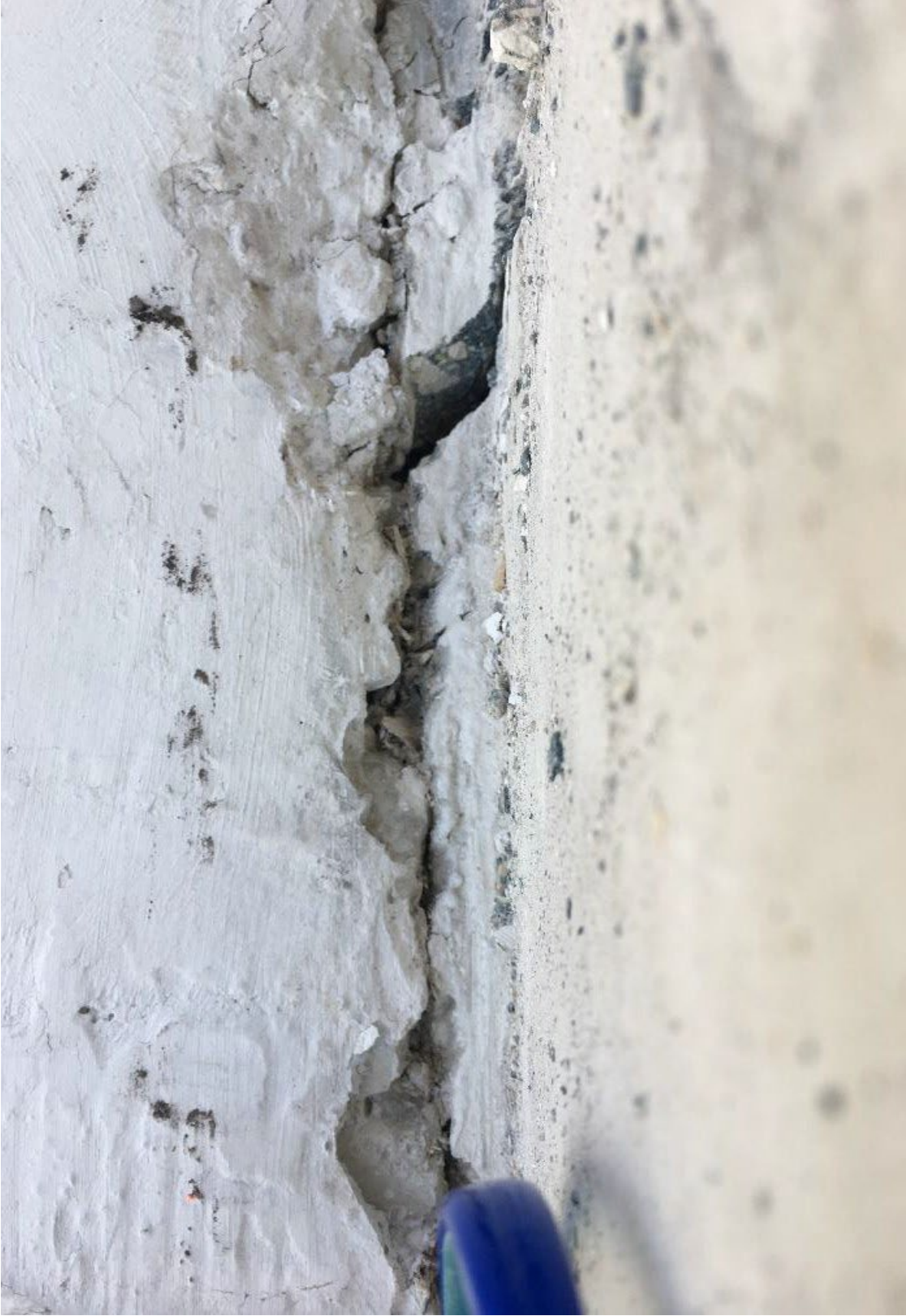
Figure 32 Cracks at the construction joint of the main span deck and diagonal 11 on 3/13/2018 by BPA
