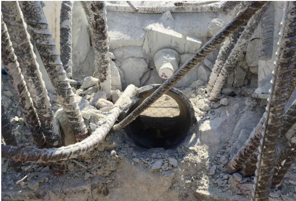
Figure 67 Punched hole in Diaphragm II at the time of the bridge collapse – from south looking towards north, April 9, 2018, by OSHA
