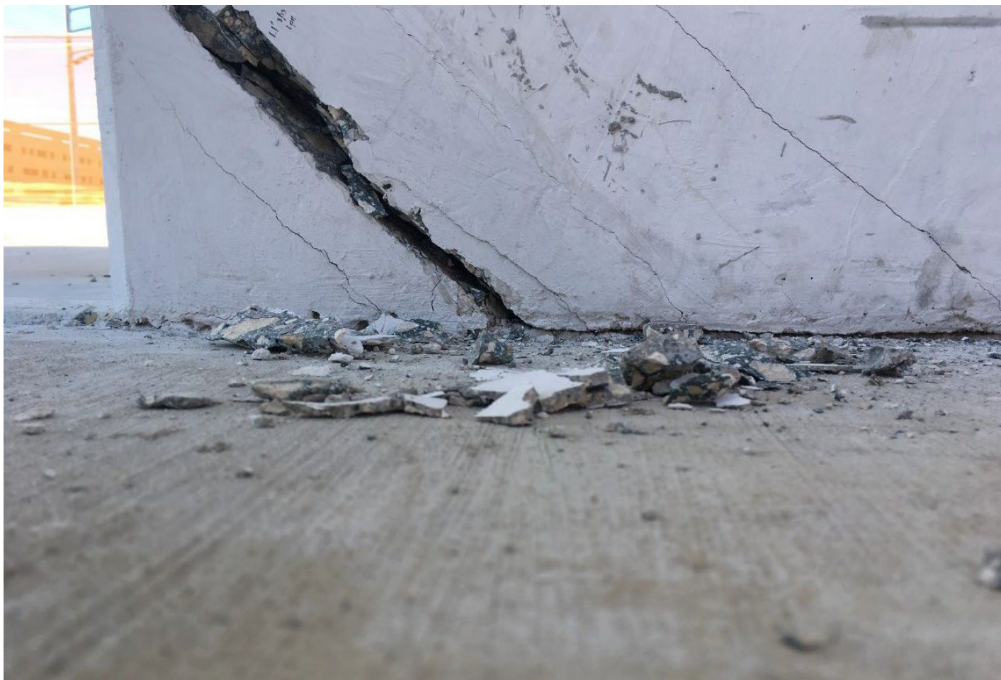
Figure 35 Cracks at the construction joint of the main span deck, diagonal 11 and the chamfer of diagonal 11 on 3/13/2018 by BPA
