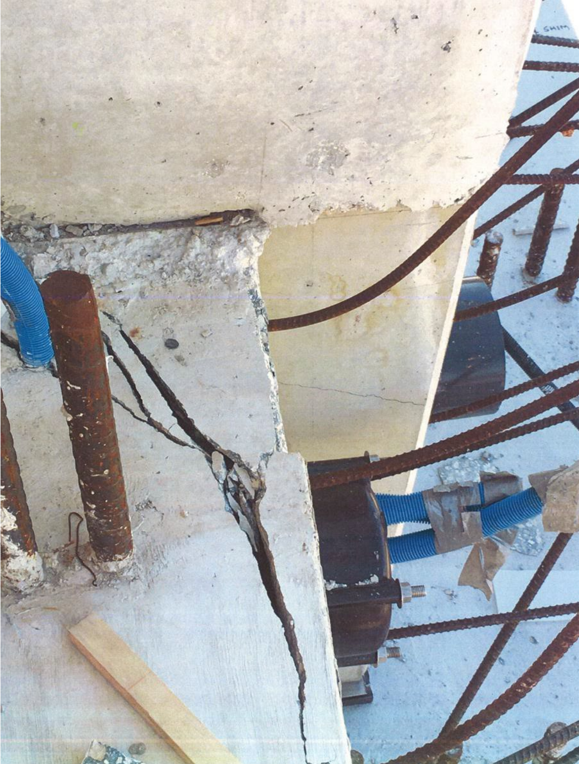
Figure 44 Cracks and movement of the column at the east side of diaphragm II on 3/14/2018 by BPA
