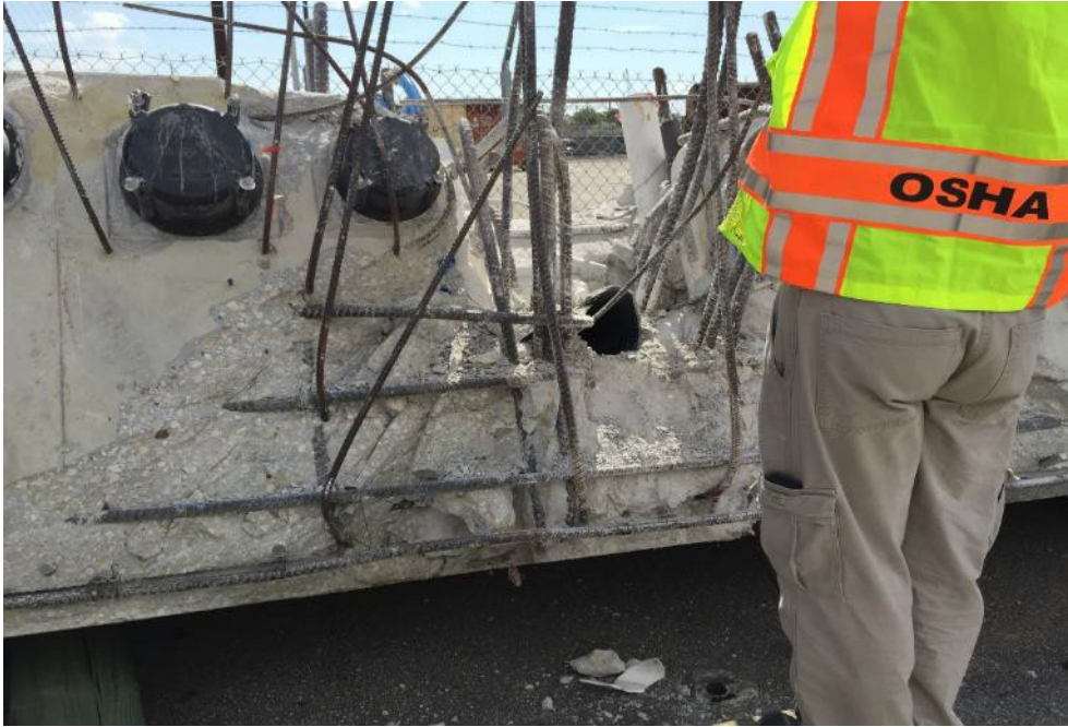
Figure 66 Punched hole in Diaphragm II at the time of the bridge collapse – from south looking towards north, April 9, 2018, by OSHA
