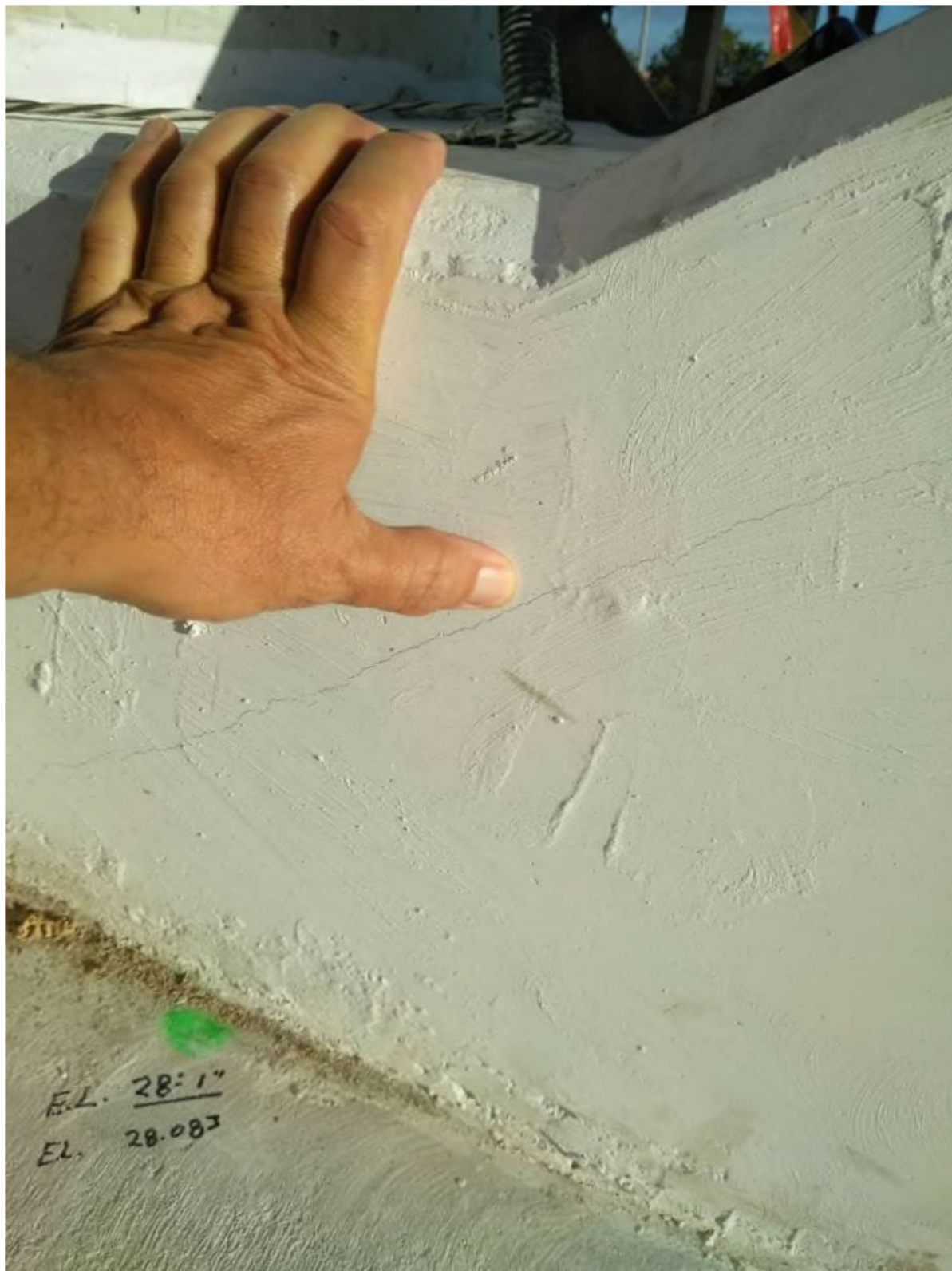
Figure 19 Photo #5 in 2/28/2018 E-mail from MCM to FIGG
