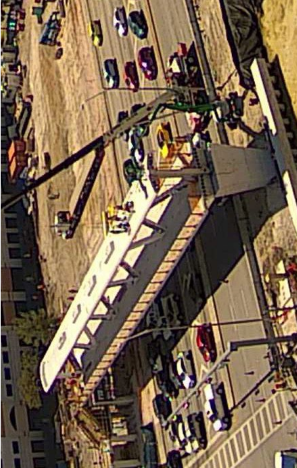
Figure 48 Bridge immediately prior to the collapse, March 15, 2018 – camera #2
