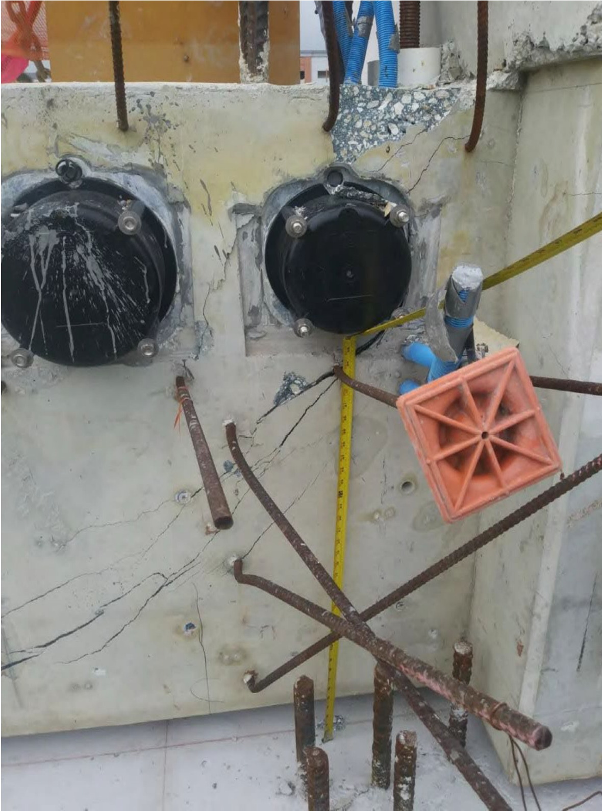
Figure 27 Cracks on the east side diaphragm II MCM email of 3/12/2018, by BPA – side face March 13, 2018 As the email was sent by MCM in the evening of March 12, 2018, FIGG did not open MCM’s email containing the photos of the cracks until the next morning on FDA, Inc.
