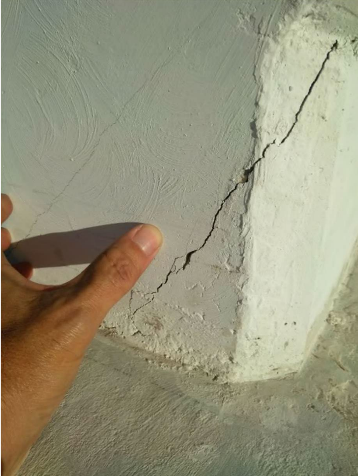
Figure 20 Photo #6 in 2/28/2018 E-mail from MCM to FIGG
