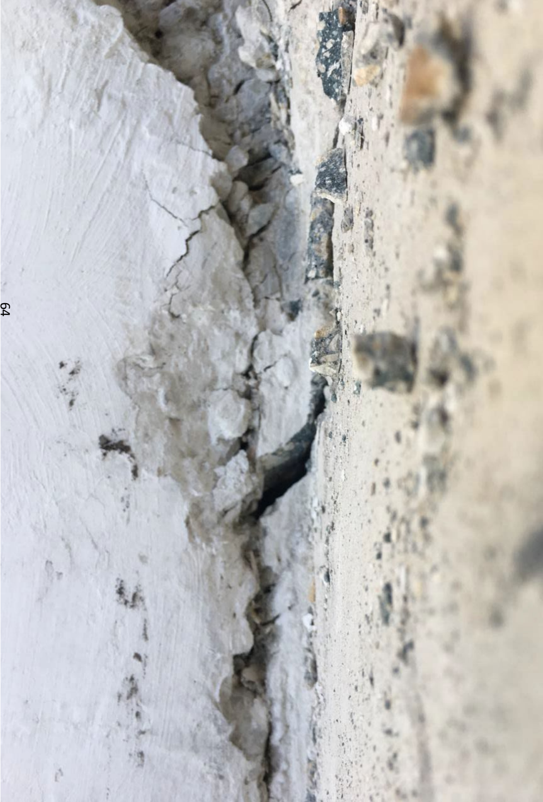
Figure 34 Cracks at the construction joint of the main span deck and diagonal 11 on 3/13/2018 by BPA
