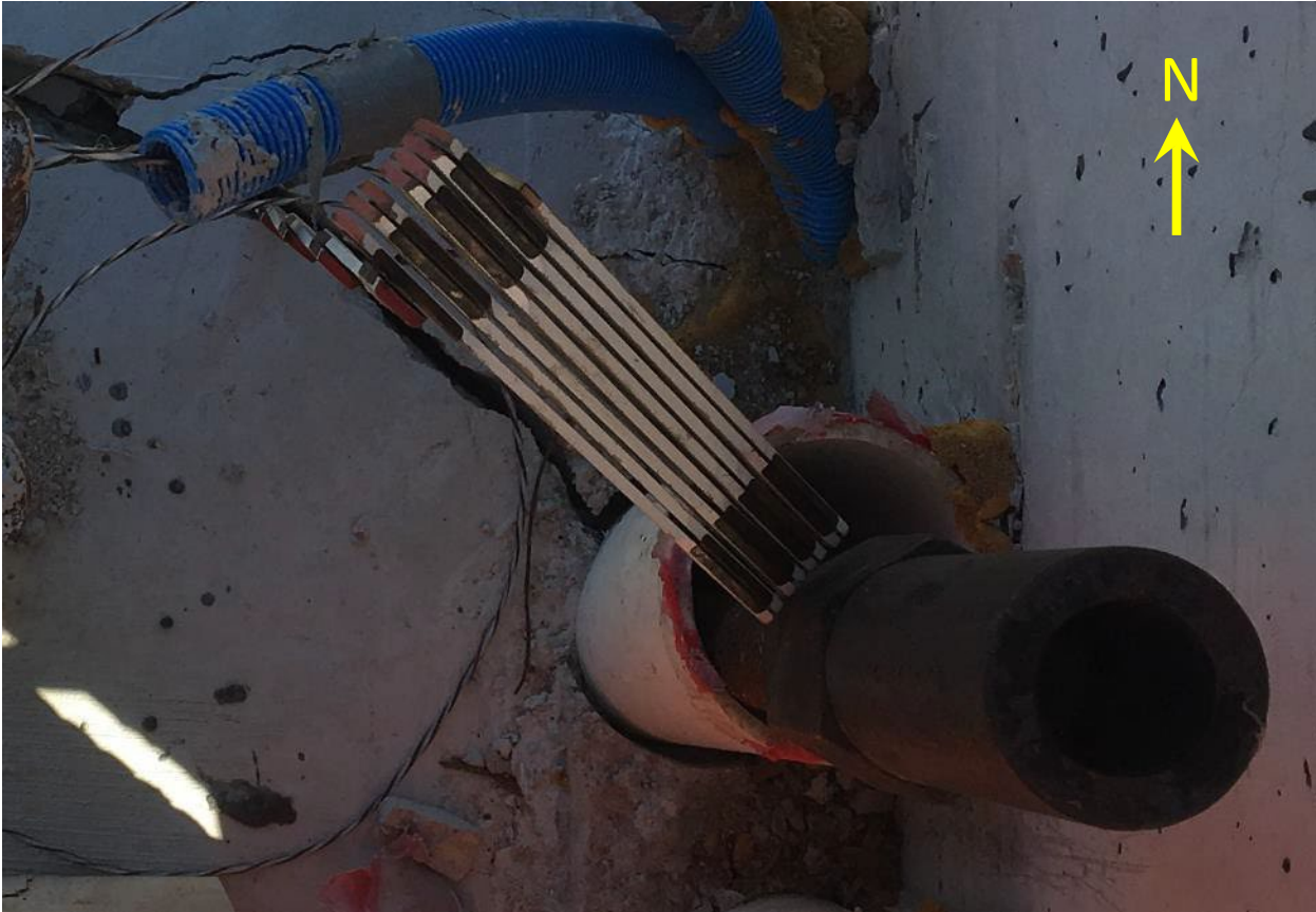
Figure 45 Note the gap indicative of movement between sleeve pipe and concrete, pictured on 3/13/2018 by BPA
