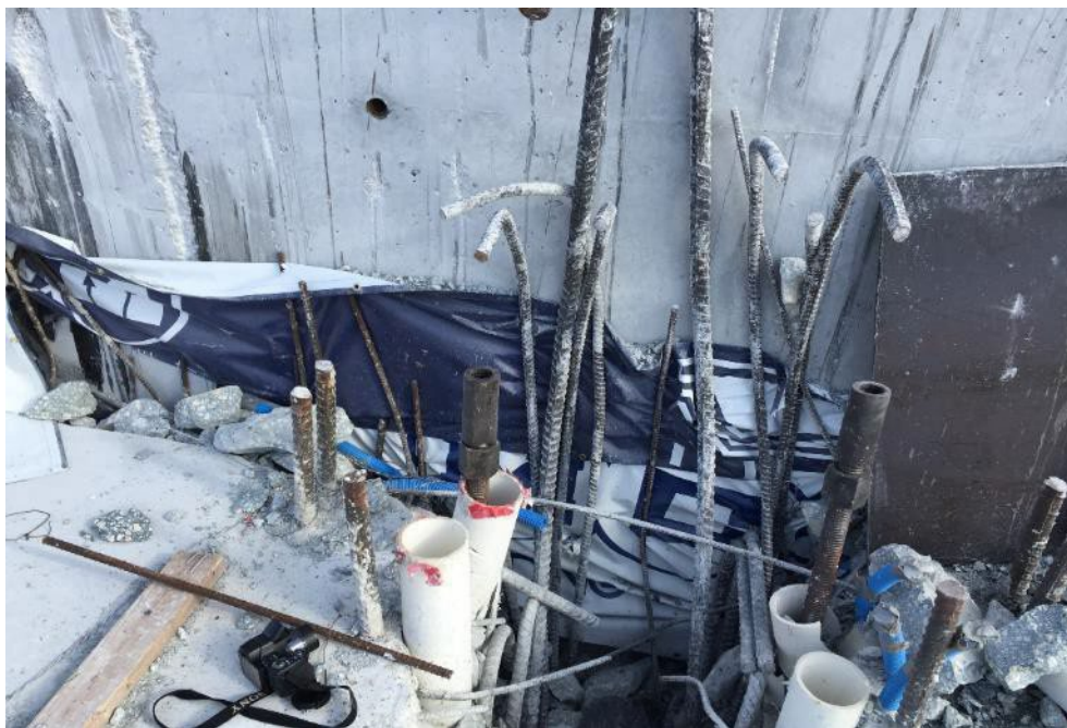
Figure 59 Concrete blow-out failure in Diaphragm II at the time of bridge collapse at the site looking north from south, March 21, 2018, by OSHA
