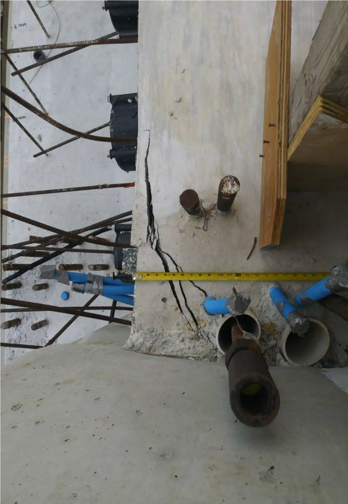
Figure 26 Cracks at the east side diaphragm II MCM email of 3/12/2018, by BPA – top face
