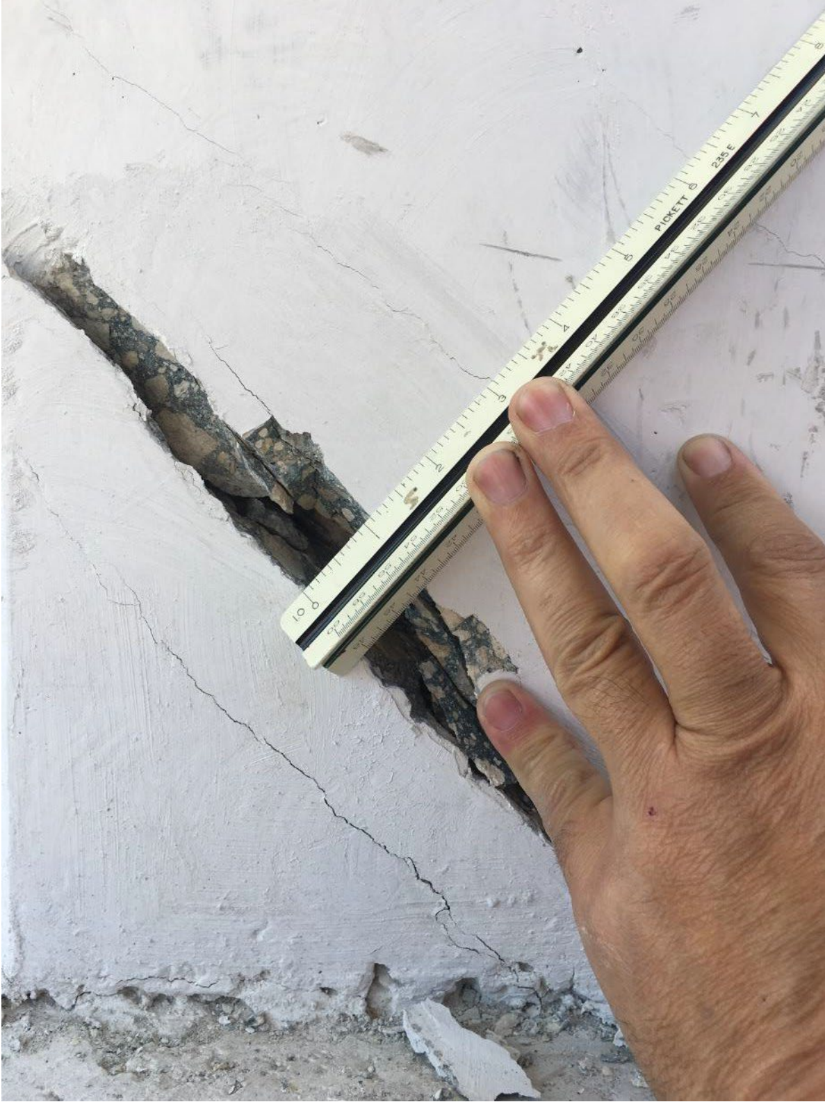
Figure 40 Close-up of longitudinal cracks in diagonal 11 on 3/13/2018 by BPA
