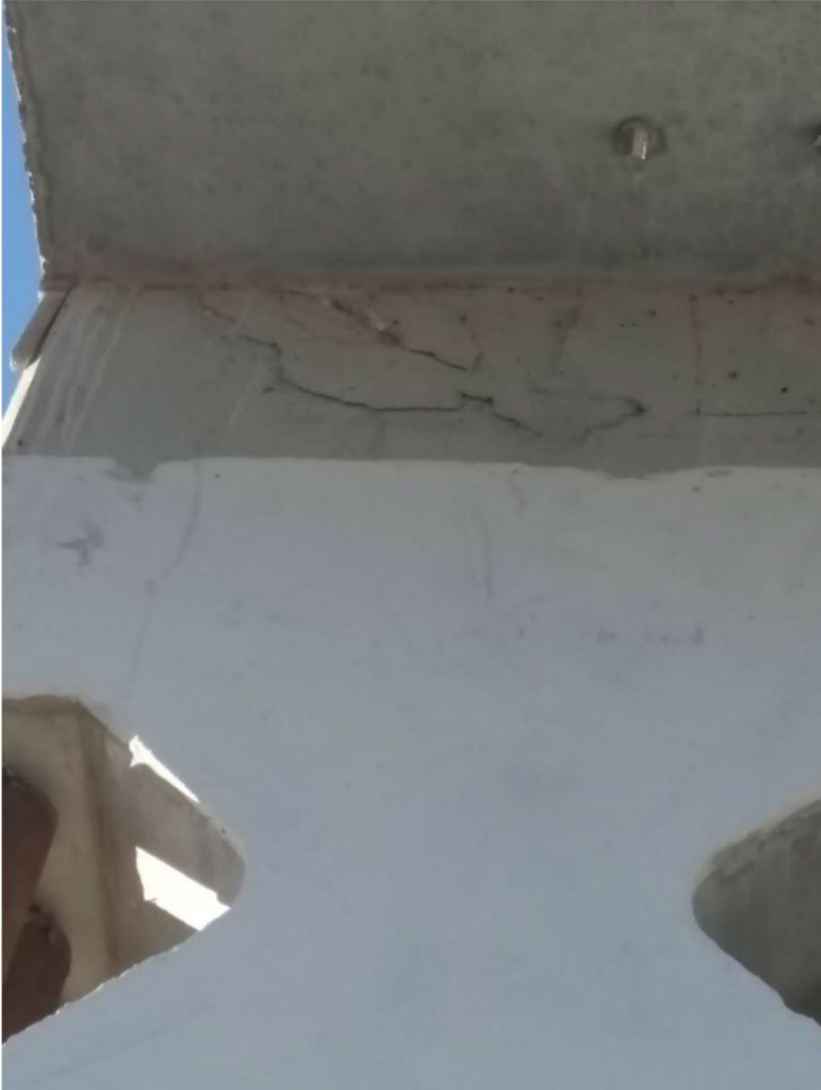
Figure 15 Photo #1 in 2/28/2018 E-mail from MCM to FIGG
