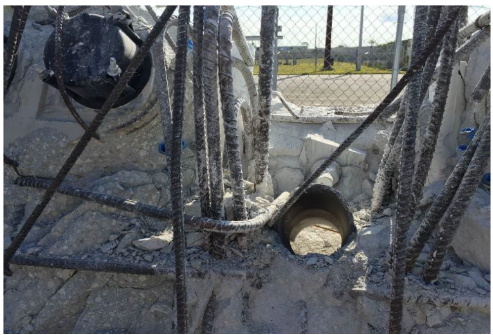
Figure 65 Punched hole in Diaphragm II at the time of the bridge collapse – from south looking towards
