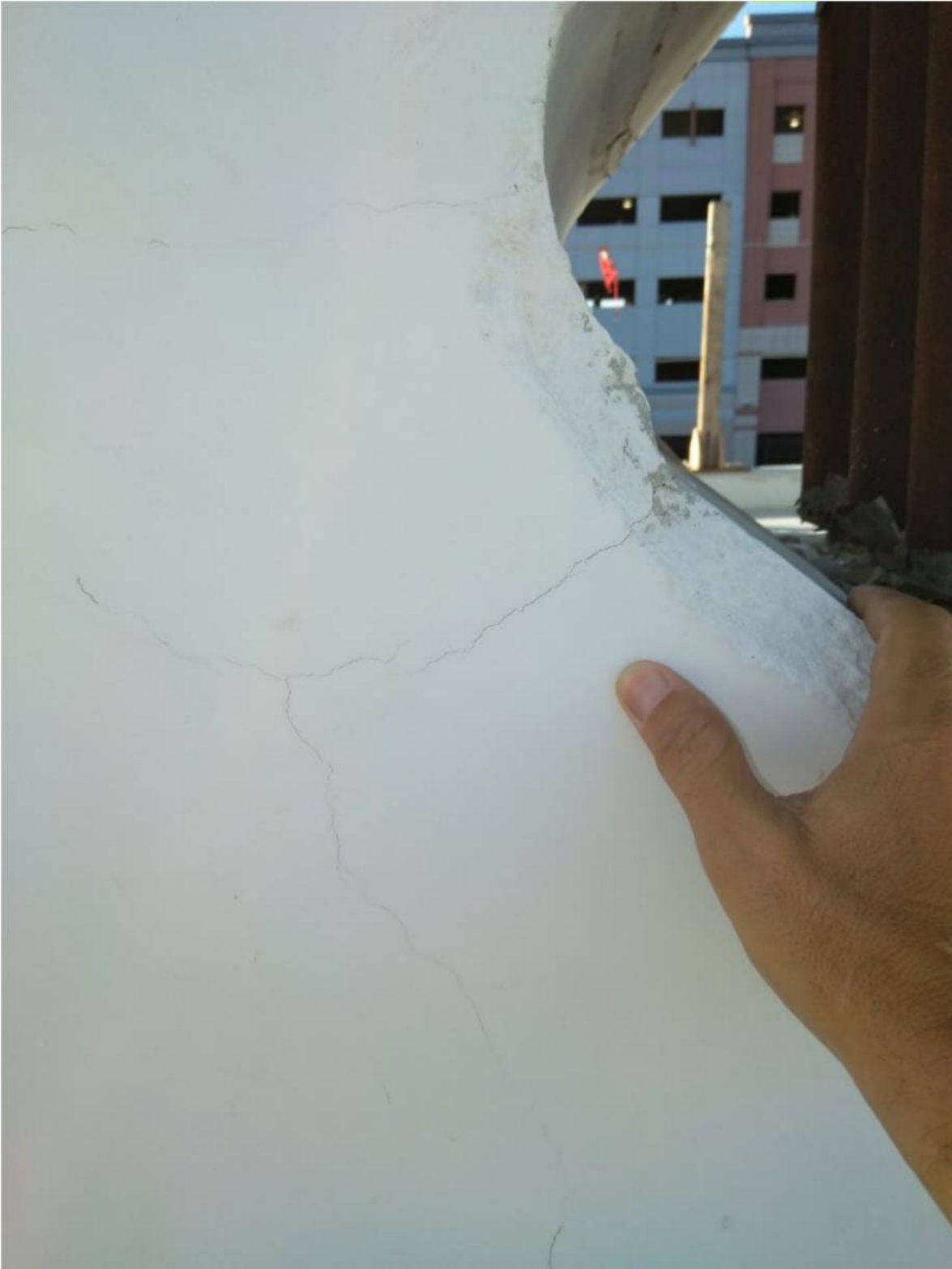
Figure 41 Photo #2 in 2/28/2018 E-mail from MCM to FIGG
