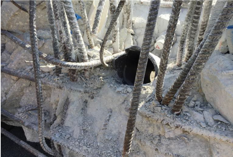
Figure 68 Punched hole in Diaphragm II at the time of the bridge collapse – from south looking towards north, April 9, 2018, by OSHA
