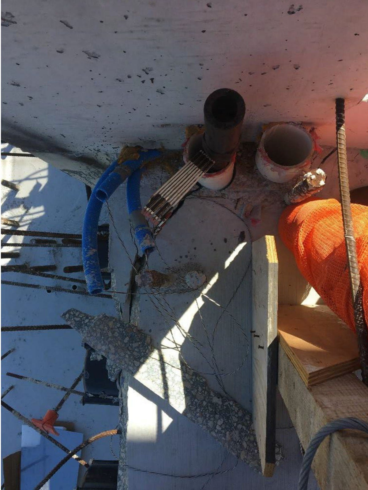
Figure 29 Close-up of cracks at the west side of diaphragm II on 3/13/2018, by BPA
