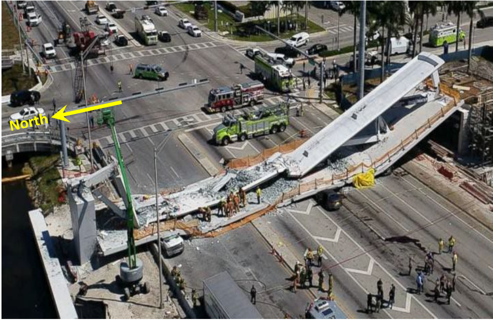
Figure 72 Aerial view of the collapsed bridge, March 15~18, 2018
