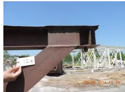
Fig. 63 – Joint 12 – West Interior
