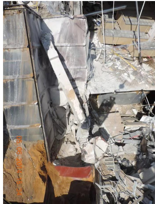
Fig. 13 NE concrete column in bin No. 1
