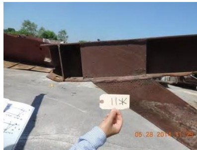
Fig. 62 – Joint 11 – West interior
