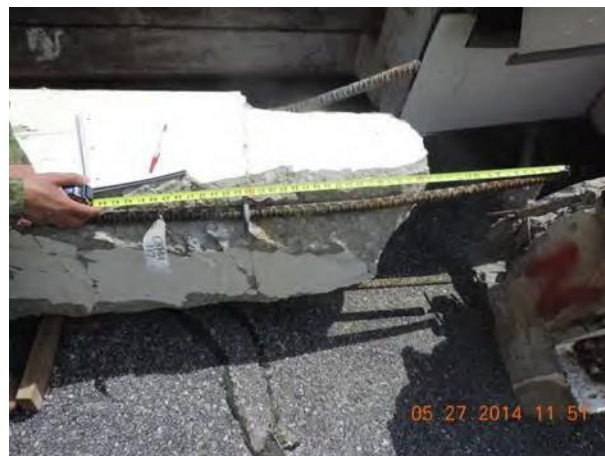
Fig. 103 NE corner column showing inadequate lap splice
