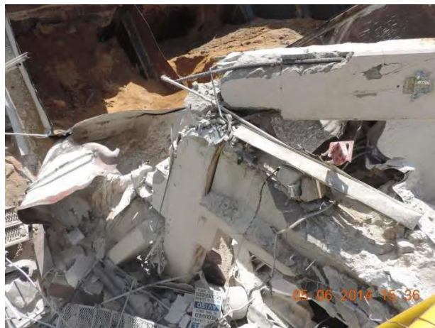
Fig. 101 Another view of fracture of NE column at 3 rd floor
