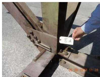
Fig. 59 – Joint 8 – West interior
