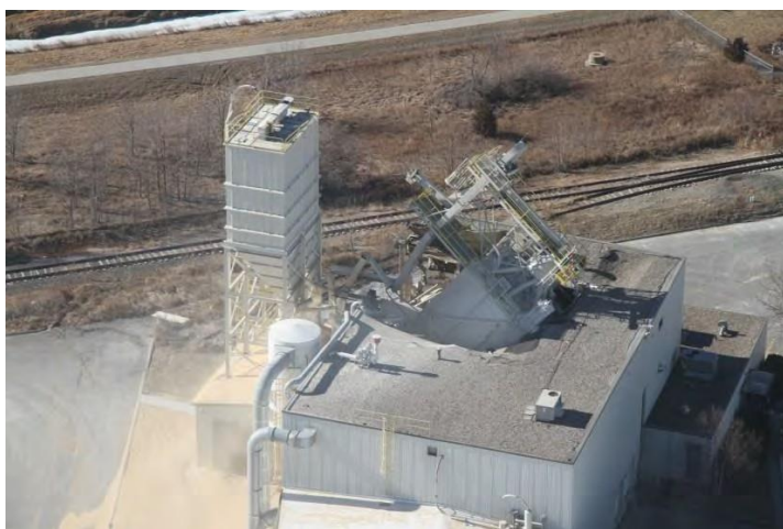
Fig. 3 Aerial view of collapse
