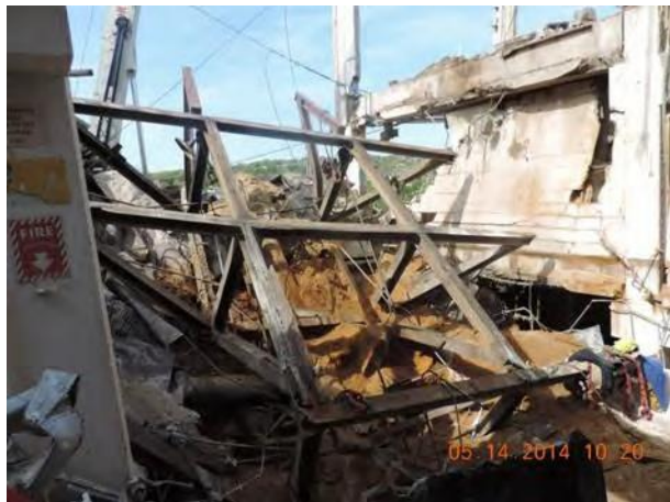
Fig. 104 Interior trusses lying in debris
