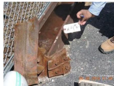
Fig. 29 – Joint 4 – South truss
