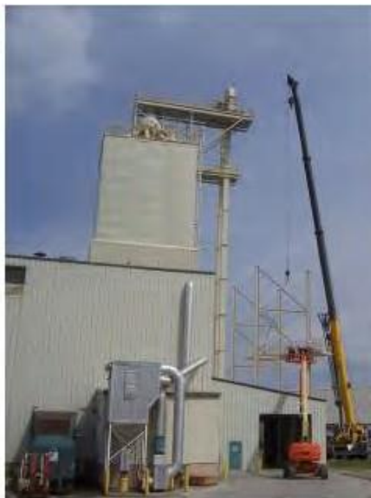
Fig. 6 Facility after modification
