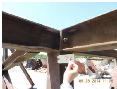
Fig. 58 – Joint 7 – West interior
