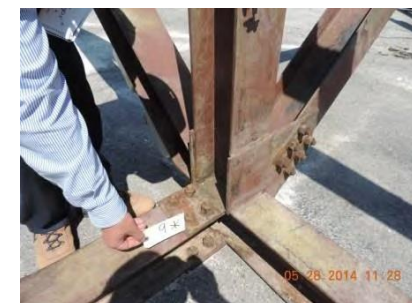
Fig. 60 – Joint 9 – West interior
