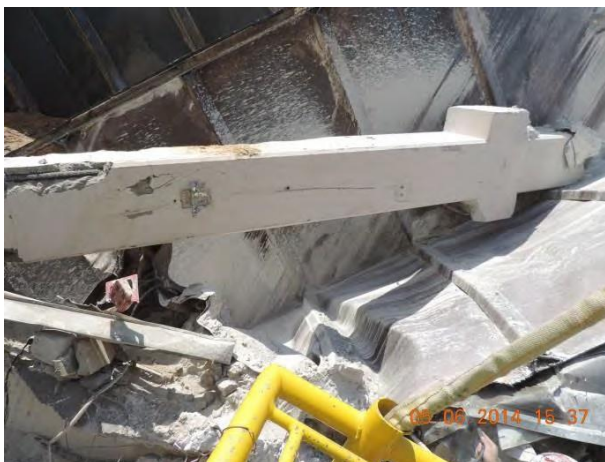
Fig. 99 – NE corner column lying in bin No. 1
