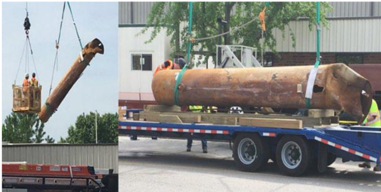
Figure 13. Removal of the SCR from Faultless Healthcare Linen facility. (Credit: CSB)
