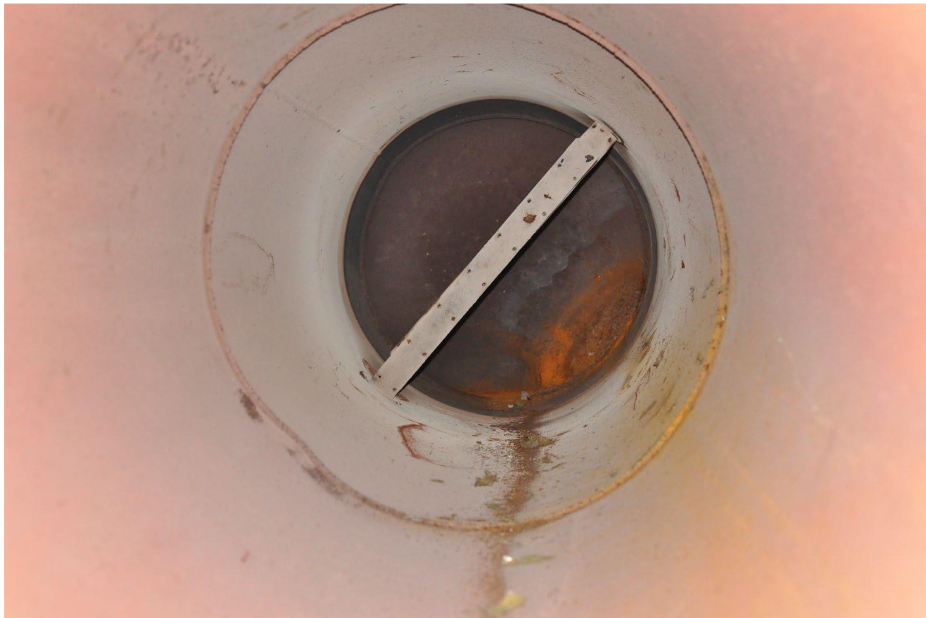
Figure 17. Photo of the inside surface of the SCR shell and upper head. (Credit: CSB)
