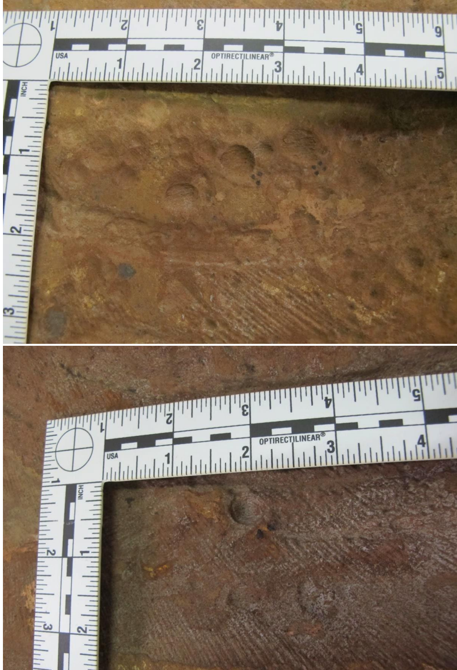
Figure 30. Pitting corrosion damage in SCR bottom head. (Credit: CSB)
