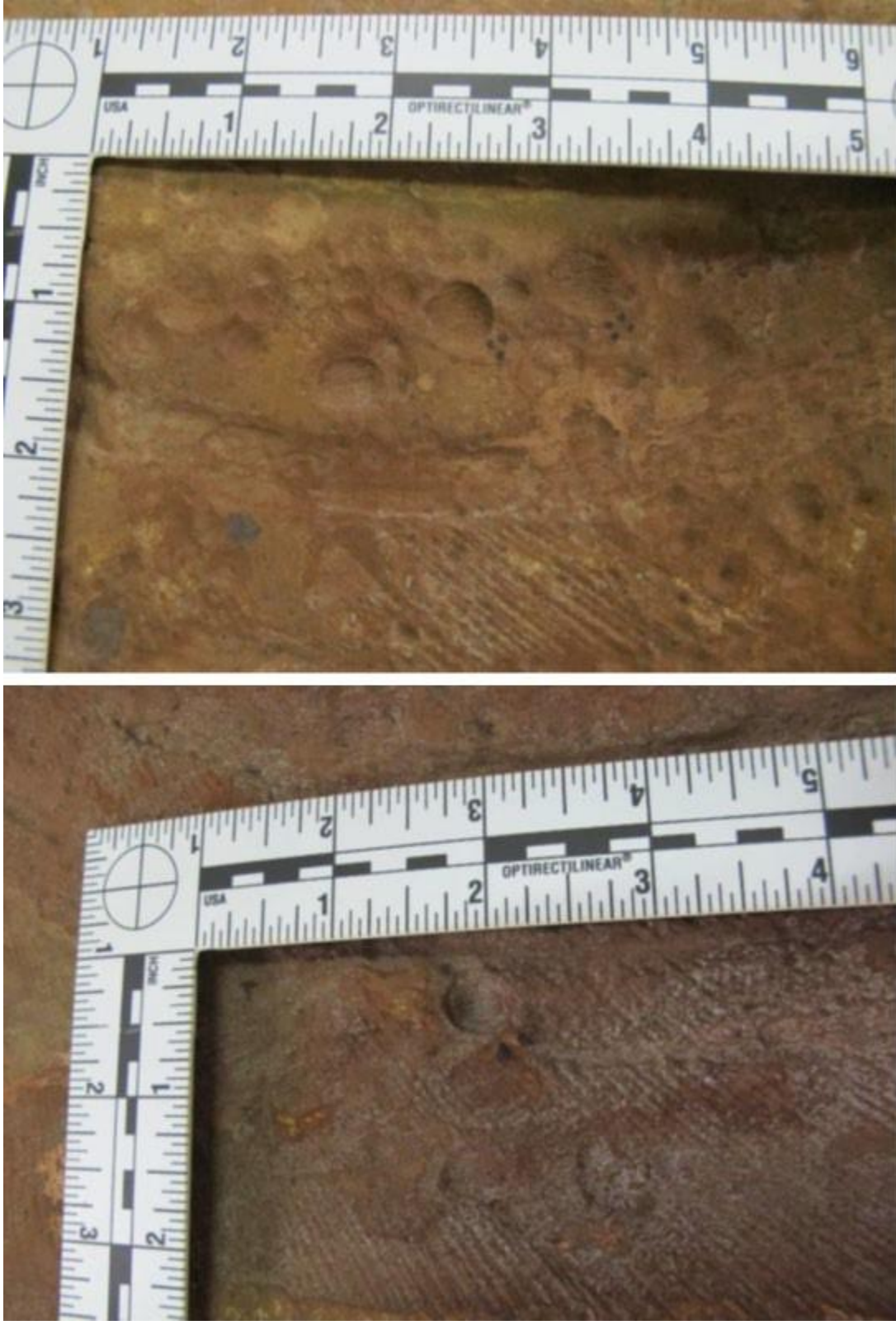
Figure 16. Pitting corrosion damage in SCR bottom head. (Credit: CSB)
