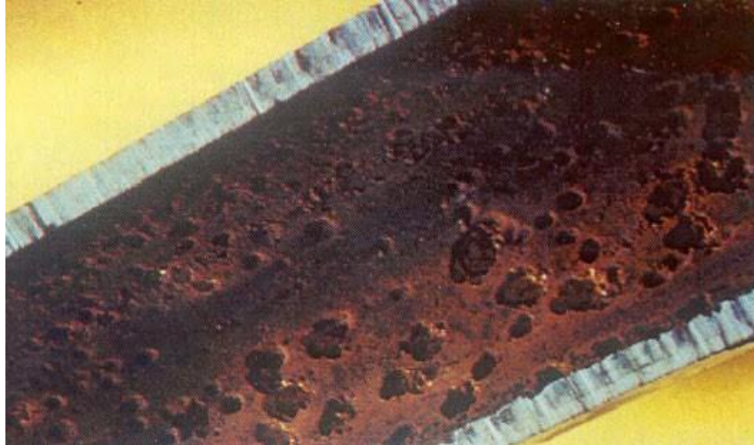
Figure 5. Pitting corrosion in a boiler tube. (Credit: U.S. Dept. of Defense [5, p. 38])
