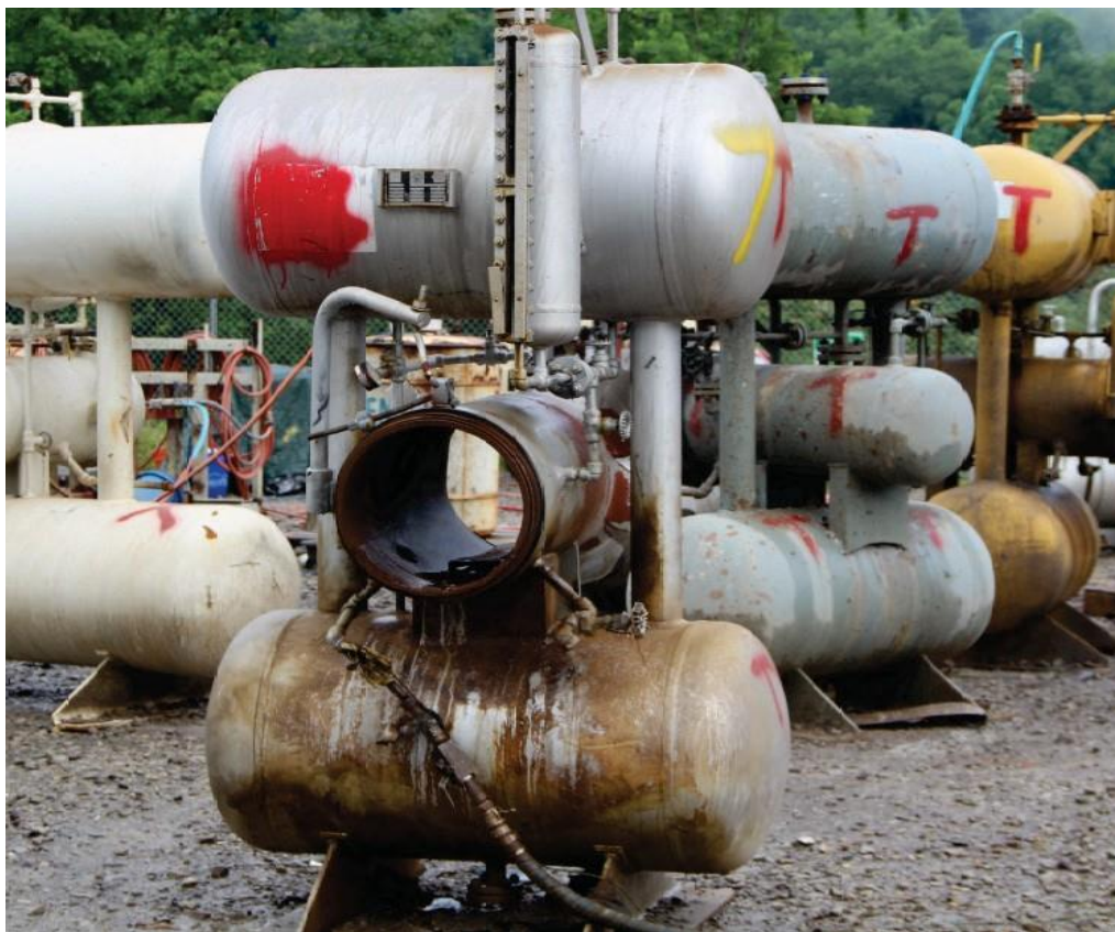
Figure 16. MP Odorizer Vessel That Exploded. This photo shows the MP odorizer that exploded on June 20, 2017. The back portion of middle chamber ruptured (see also Figure 17) and the front threaded section blew off. The aluminum tray and mechanical parts that were inside the middle chamber were expelled from the MP during the event. (Credit: SPSI).
