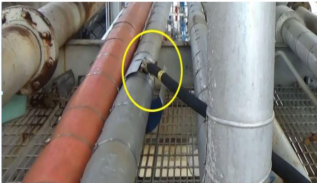
Figure 30. Hot Water Hose Positioned on the Liquid Methyl Mercaptan Feed Piping. Hot water flowed between the piping and the insulation to heat the piping and dissociate the solid hydrate that had formed after water inadvertently entered the methyl mercaptan storage tank. Source: CSB.
