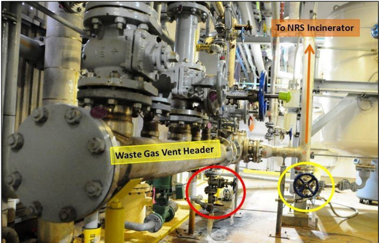
Figure 2. Waste Gas Vent Header Piping on the Third Floor of the Manufacturing Building. This portion, where several waste gas sources come together, is referred to as the waste gas vent header . Waste gas from this portion of the vent header traveled up to reach the NRS incinerator, a piping configuration that created a low spot where liquid accumulated. To remove the liquid during waste gas vent header piping high-pressure events, operators were instructed to open valves (yellow circle) and drain the system through a hose routed to a floor drain located near a safety shower. The floor drain is connected an open trench-type sump on the first floor. At the time of the incident, a second set of drain valves (red circle) were also opened directly to the floor inside the manufacturing building. Source: CSB.
