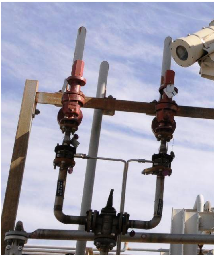
Figure 33. Nitrogen Relief Valves at One of the Two Methyl Mercaptan Railcar Unloading Stations. DuPont PHAs and relief valve design documents never considered the possibility of lining up the methyl mercaptan storage tank pumps to these relief valves—as they were at the time of the incident. As a result, liquid methyl mercaptan was discharged from a system designed for nitrogen vapor. Source: CSB.
