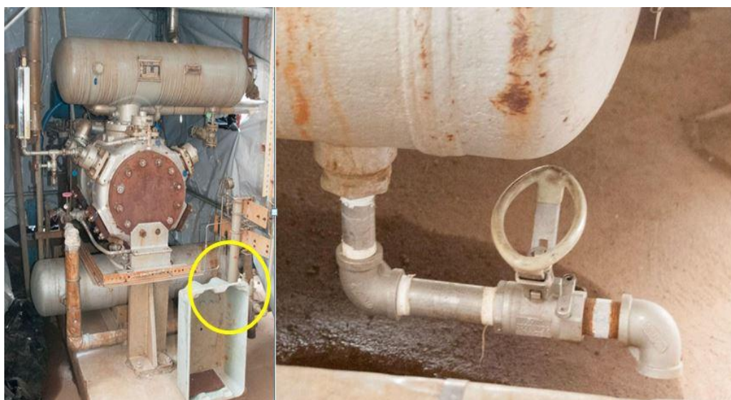
Figure 38. Methylene Chloride a Compressor. Photo shows where operators routinely drained liquid accumulation from a methylene chloride compressor without using line-breaking procedures. Source: CSB.
