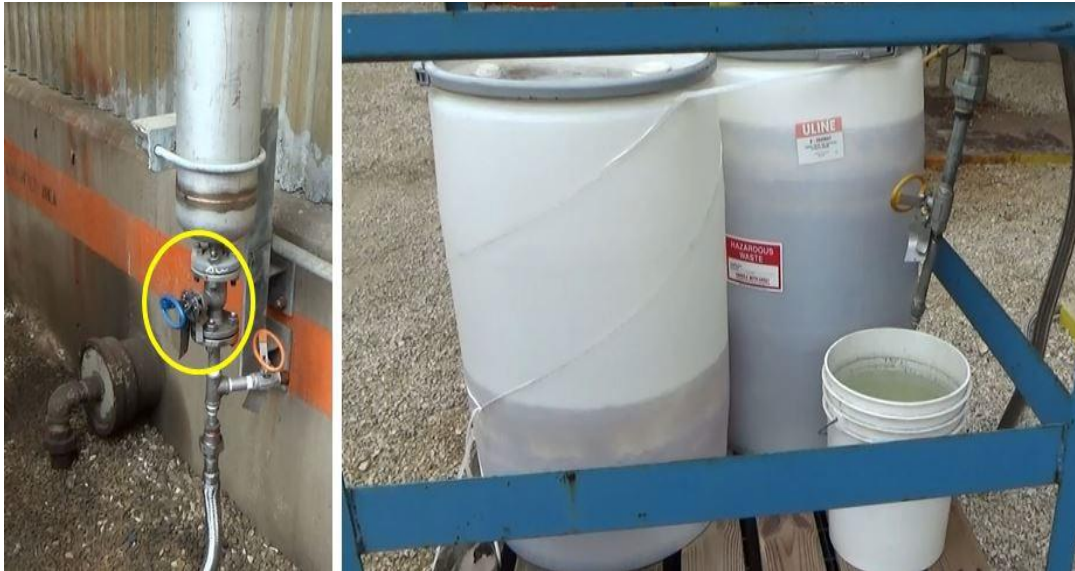
Figure 37. Photo Showing Another Line Break. Operators drained liquid accumulation in another vent header without using line-breaking procedures. Source: CSB.
